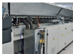
Maintenance "On-the-Fly" continues to operate while the condensation management system is being cleaned
